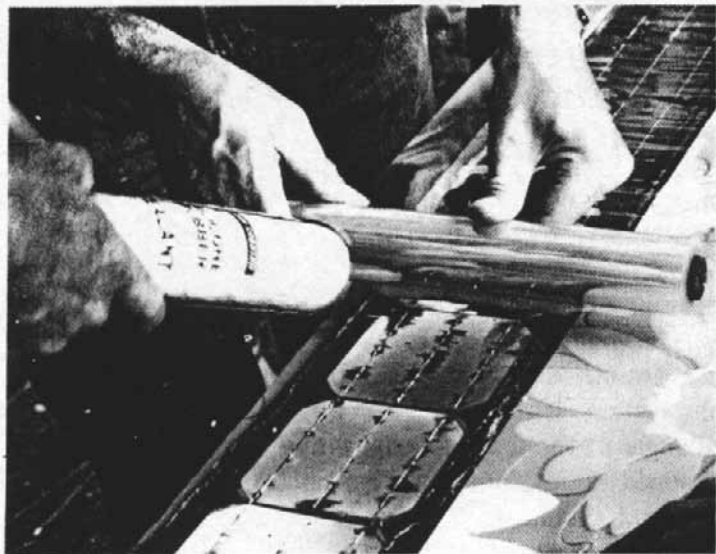
FIGURE 4.12—Coating the top of the cells with silicone and Mylar film. The Mylar film squeezes out a bead of the silicone RTV, eliminating voids and air bubbles (Courtesy Home Energy Workshop, Fort Collins, Colorado).
