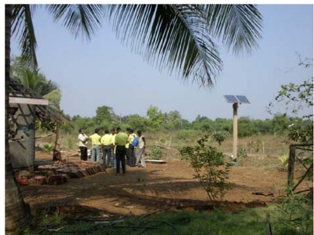
Fig 7 Cottage industry group in India installing a pole mount PV system at a “green” resort near Mumbai.
