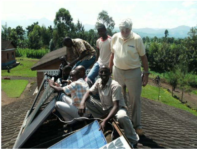
Fig 8 Richard Komp helping the Radiant Horizon group find the problem (a broken wire) on a non-functional PV array on a health clinic in Rwanda.
